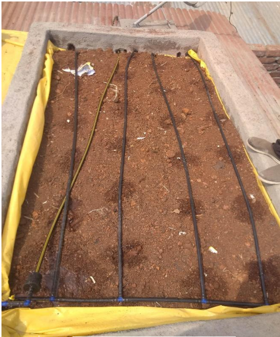
Rooftop Garden Irrigation System
