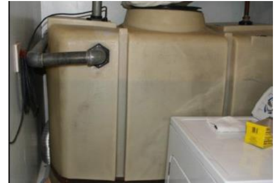
Indoor Water Storage Tank w/ Submersible Pump
