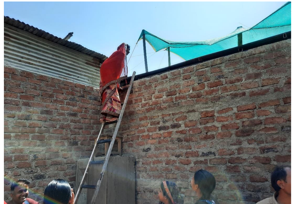
Resident climbing the ladder to look at the rood top garden during 'Experience Tour', Pune.
