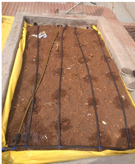
Rooftop Garden Irrigation System
