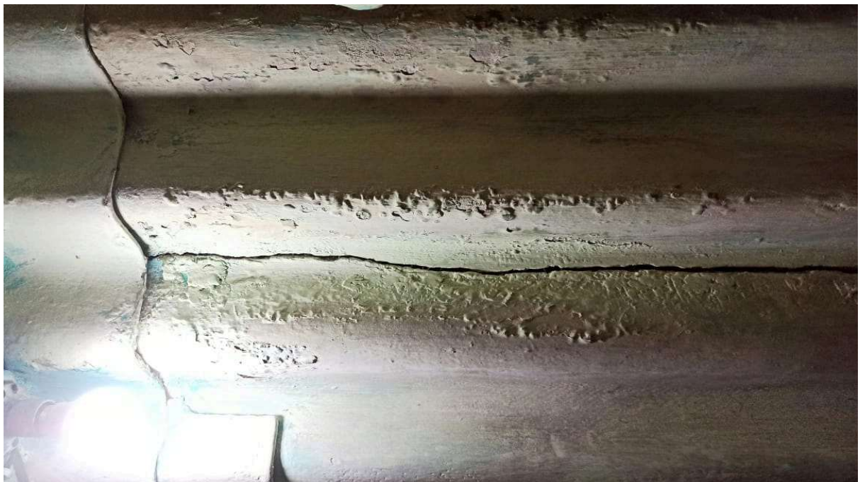
Fig 25.2.1.7-1 : Crack in the Roof
