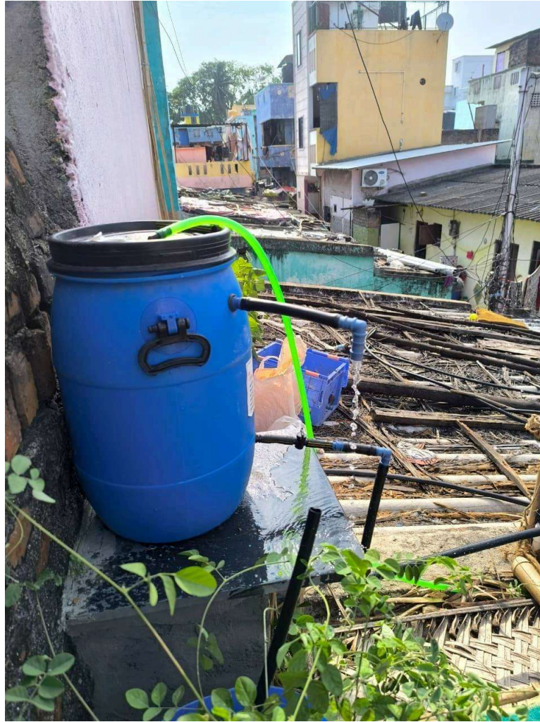
Fig 37.4.2-18 : Water over flowing through the Tank's outlet
