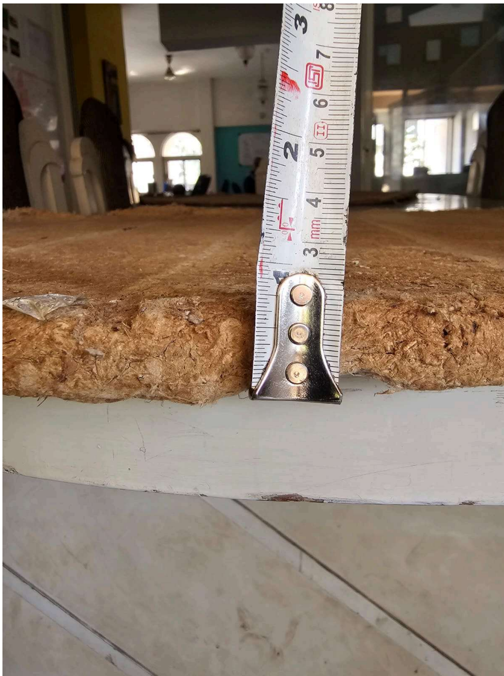
Fig 37.2.3-5 : Check if panel thickness is at least 15mm and there is uniformity in thickness
