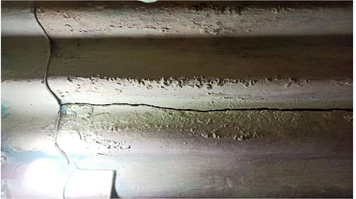
Fig 25.2.1.7-1 : Crack in the Roof
